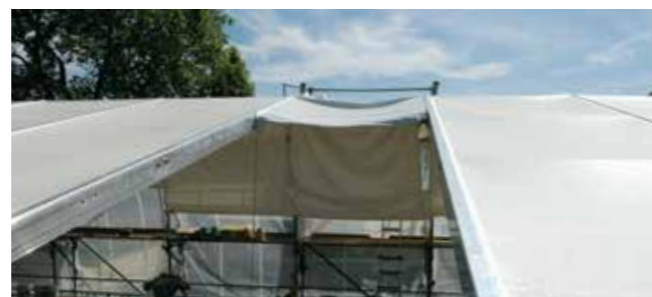
Temporarily open "empty bay" for servicing the site; the gaps between the frame sections are also very suitable for equalisation in a longitudinal direction
