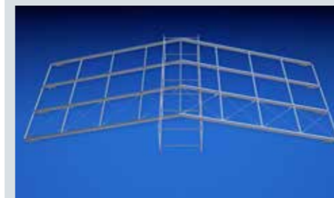
Pre-assembly of a three-section field on the ground (a temporary support structure out of scaffolding material in the middle)
